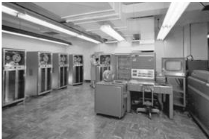
Typical air con Room with mainframe computer.
